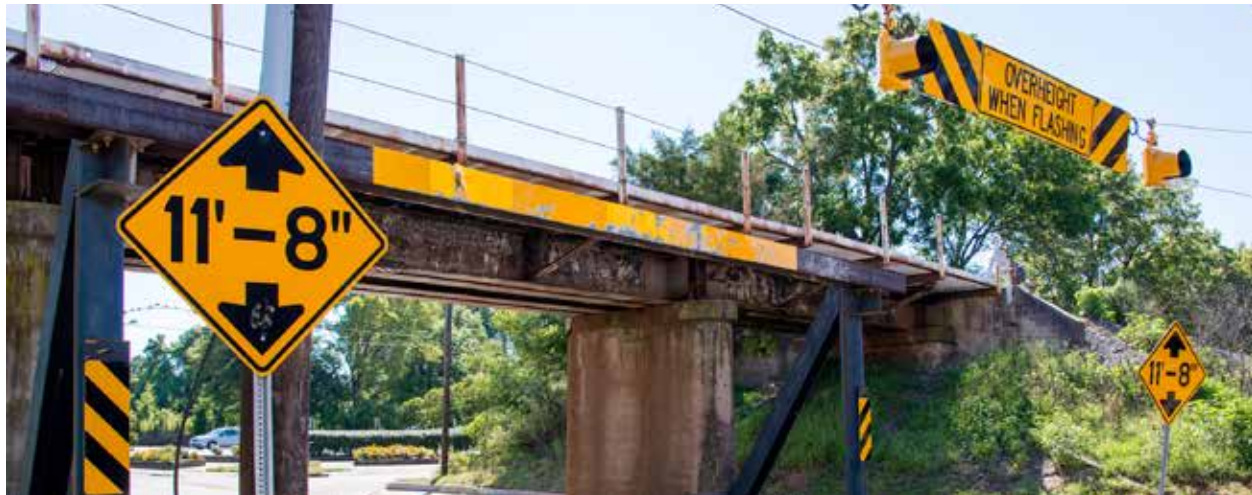
The Gregson Street Bridge with the previous overheight detection and warning system. Source: Washuotaku, Wikimedia Commons, licensed under the Creative Commons Attribution-Share Alike 4.0 International license.
