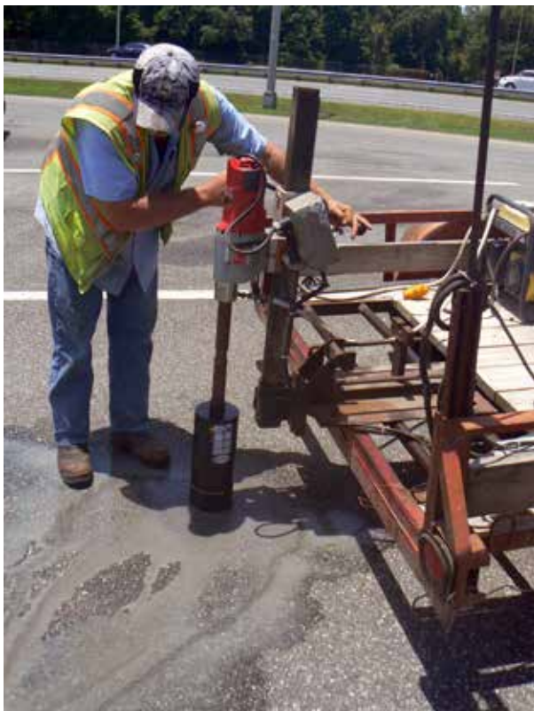
Installation of TPAS technology. Source: FDOT.
